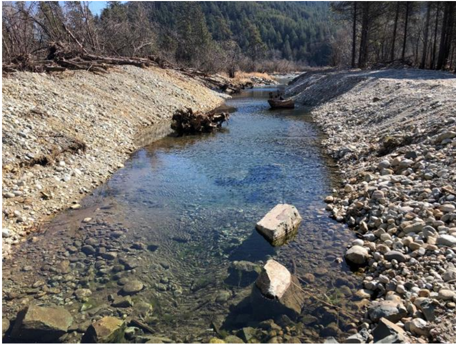
Photo 1 Looking south along William Phillips at typical new channel construction conditions; large woody debris placement installed (March 16, 2020).
