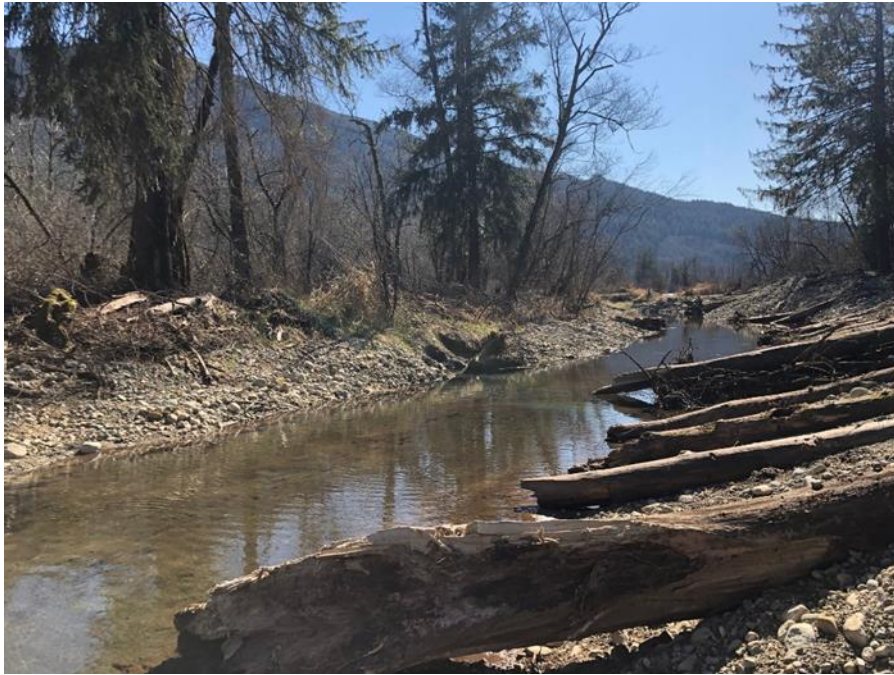
Photo 1 Looking south along Nancy Phillips west bank at typical new channel construction conditions; large woody debris placement installed (March 16, 2020).
