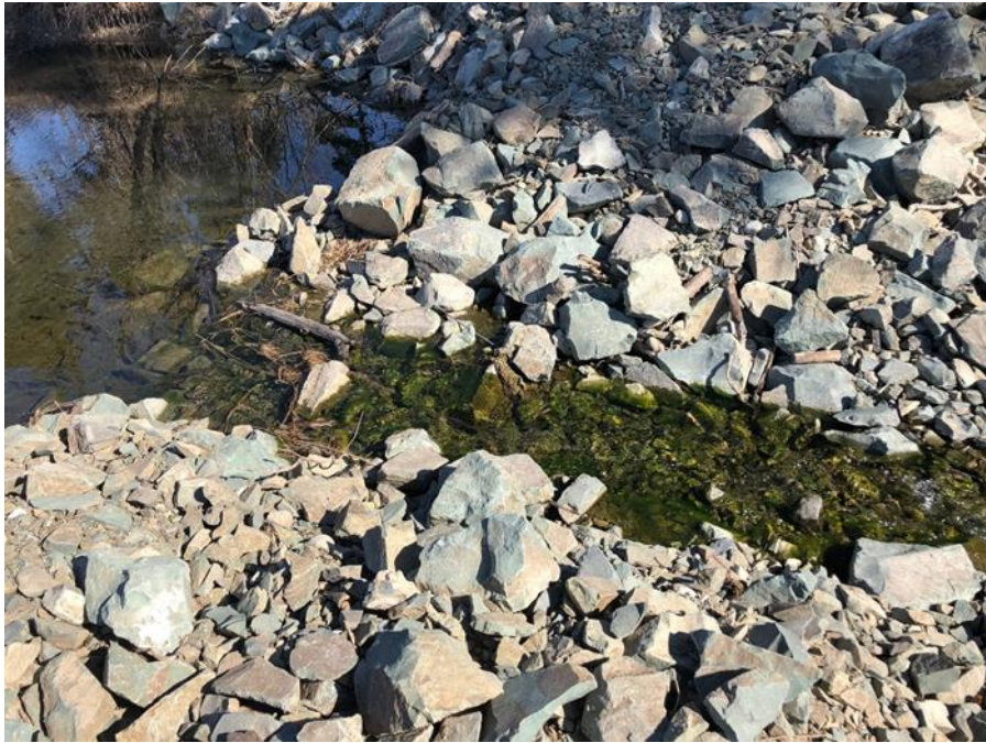
Photo 7 Looking north at William Phillips Slough Weir 1B closest to the Harrison River confluence (March 16, 2020).
