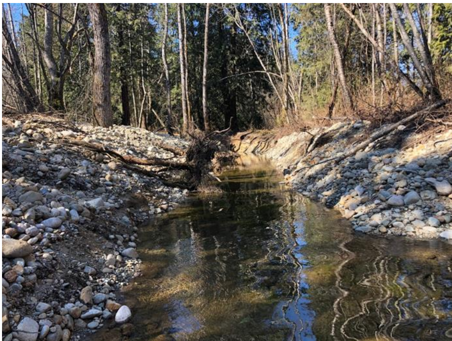
Photo 2 Looking north along the new constructed channel of Nancy Phillips Slough at typical bank conditions (March 16, 2020).
