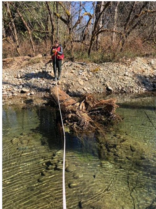
Photo 6 Large woody debris structure installed in Nancy Phillips Slough and functional (March 16, 2020).
