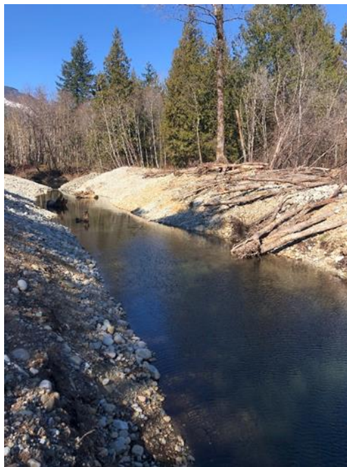
Photo 2 Looking north along the new constructed channel of William Phillips Slough at typical bank conditions (March 16, 2020).
