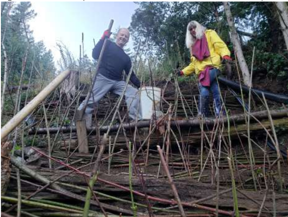
Figure 8. Volunteers install bioengineering wattle fence at active bank erosion site on lake foreshore.
