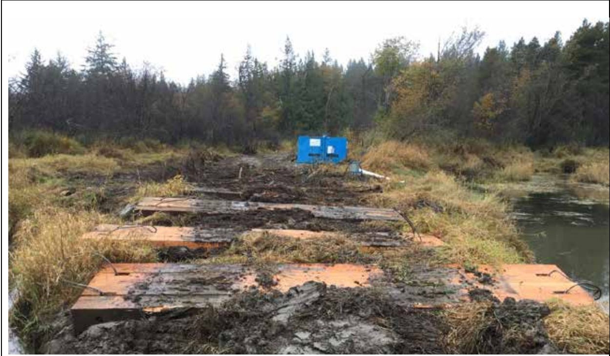
Photo 3 October 17, 2019 – Swamp mats laid out for machine access on William Phillips Slough.
