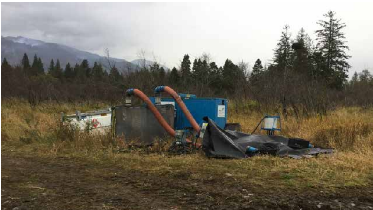
Photo 2 October 15, 2019 – Pumps used for dewatering of the work area at William Phillips Slough.
