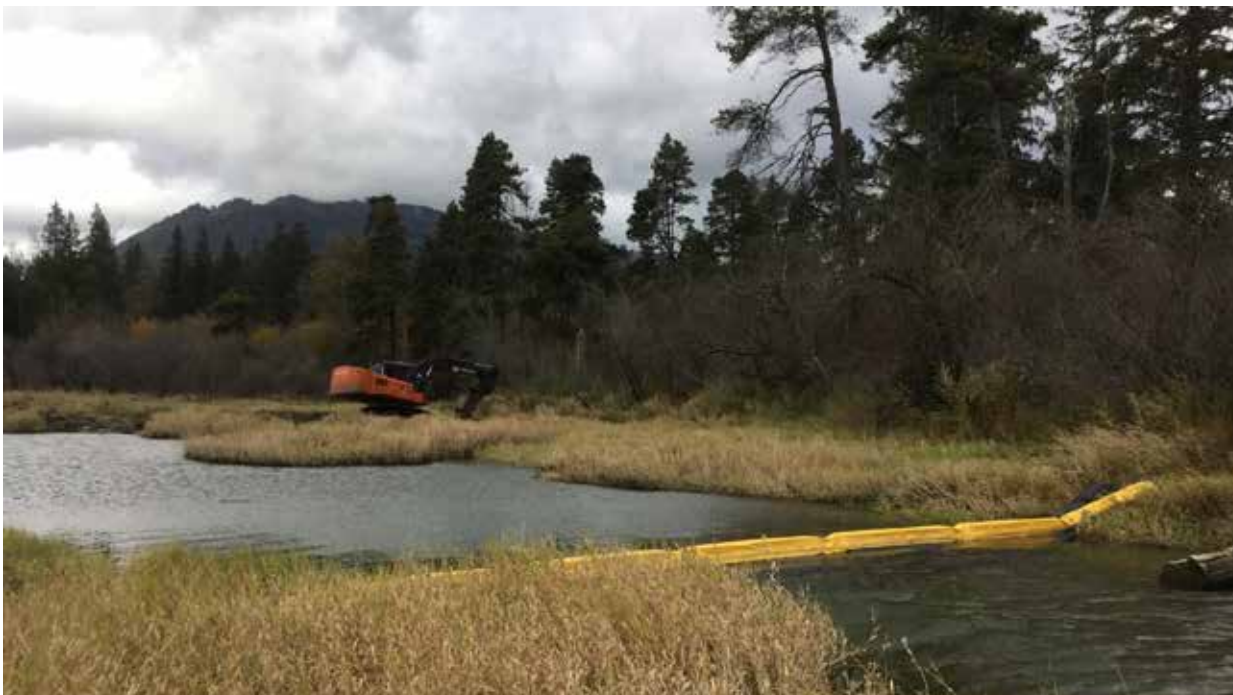
Photo 8 October 25, 2019 – Silt curtain at downstream extent of the William Phillips Slough to isolate work area.
