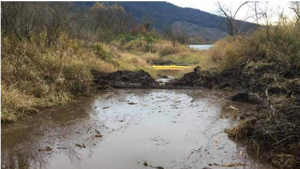
Photo 14 November 7, 2019 - View of earth berm and silt current used to isolate the construction area at Nancy Williams Slough.
