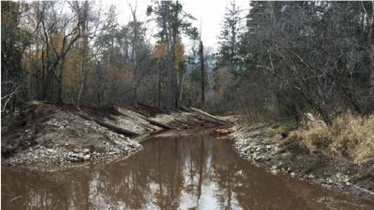
Photo 13 November 7, 2019 - North view of construction channel near the north end of Nancy Phillips Slough.
