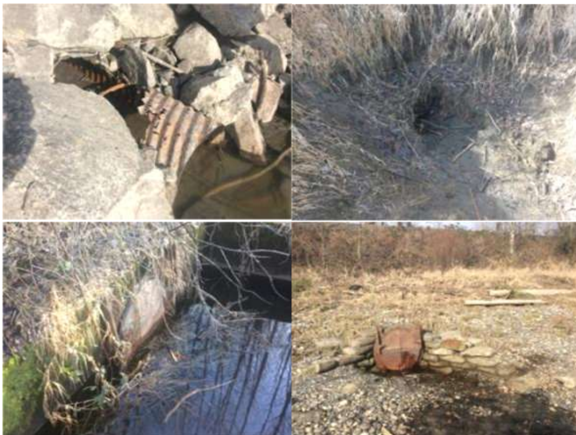
Figure 4: Access barriers to Sq'ewlets Slough East (Top), Sq'ewlets Slough West (bottom left) and Sq'ewlets Marsh (bottom right) on February 10, 2020.
