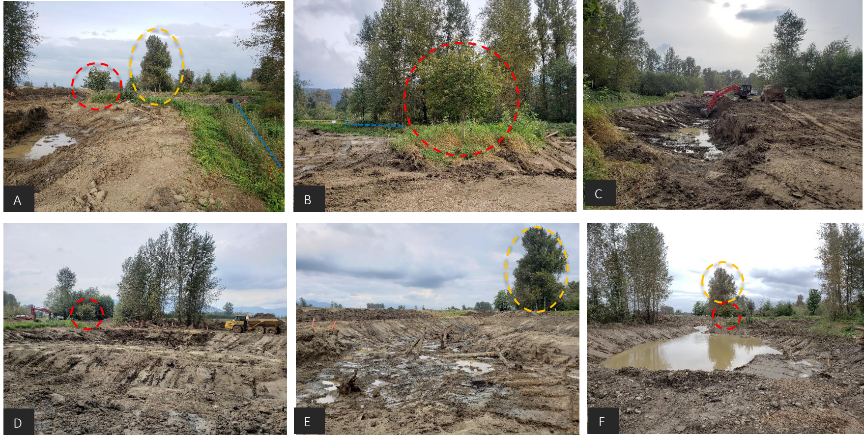
A. 2019 Instream east view with two reference tree clusters (red polygon and yellow polygon) during construction, with 2018 instream channel creation indicated as blue dashed line. B. south-east view of wetland construction. C. West-view of connection channel from wetland to constructed stream (2018). D. North view of wetland during construction. E. North-east view of wetland construction F. East view of construction, prior to LWD placement, and after groundwater has been exposed.
