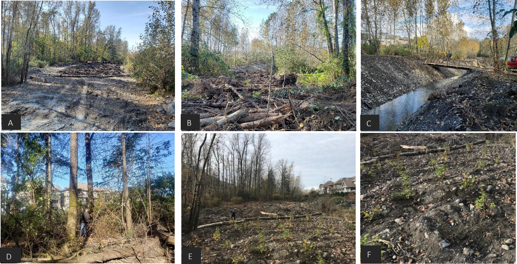
A. Downstream view machine roughening and loosening soil to reform floodplain forest. B. Rootwads and logs added to support soil and forest regrowth and close access. C. Footbridge required to reconnect trail. D. Hazard tree risk assessment. E. FVWC plants access with native plants. F. Close up of native plants being dug-in.
