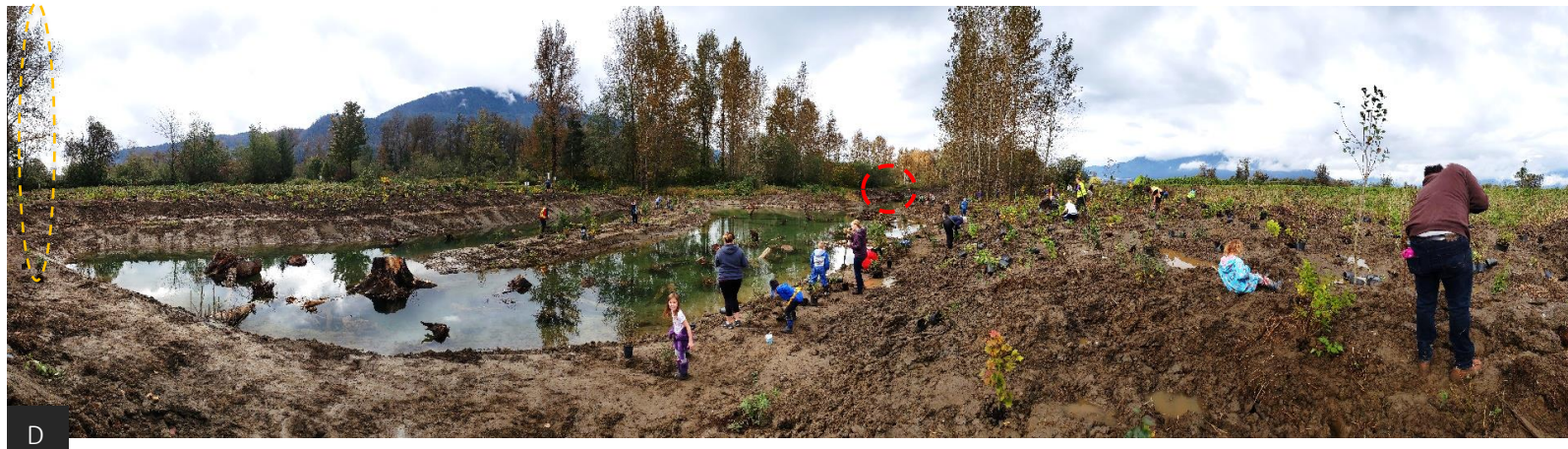
A. Intake pipe and flange from 2018 instream and the connection pipe to supply wetland with summer flows. B. East view of wetlands after rootwads installed. C. Volunteers planting. D. Panoramic view of volunteers planting.
