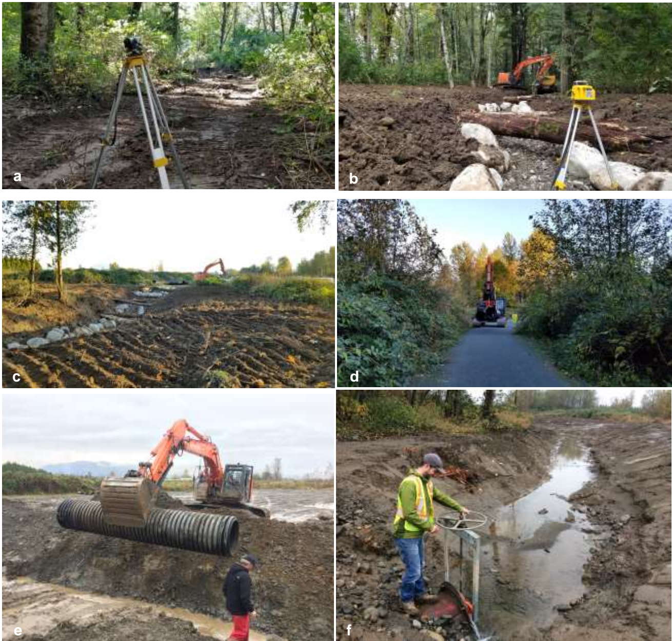
Figure 1. Photo-documentation of the instream restoration works. A. Alignment roughed out and surveyed. B. Construction of channel alignment, with boulders along bank to protect fine substrate from sloughing. C. Construction along alignment near Hooge Rd parking lot. D. Contracted flagger-mobilizing machine down dike infrastructure, ensuring public safety. E. Installation of PVC pipe to support conveyance of water at Hooge Rd parking lot. F. City staff worker opens the control valve at upper end of Peach- connection channel Nov. 2018.
